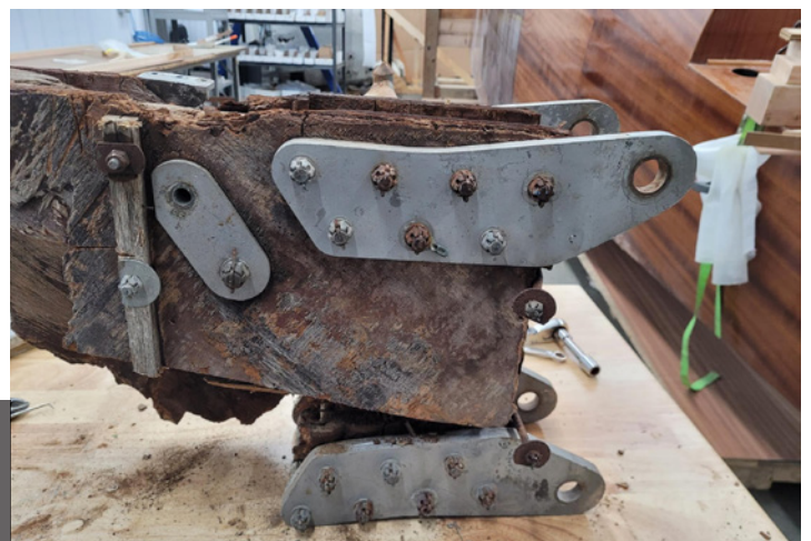
A closer view of the original attach plates.
