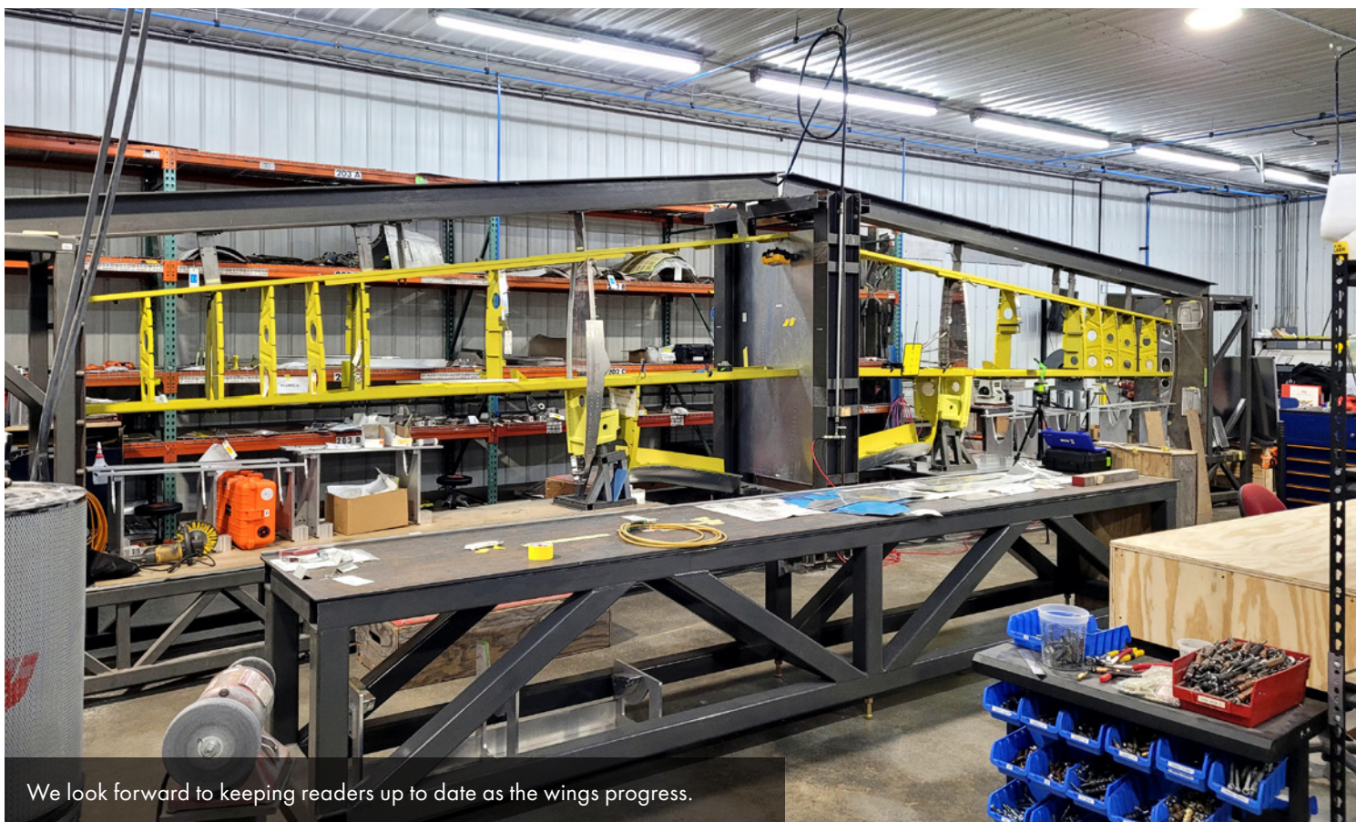
More and more ribs are installed as the wings continue to take shape.
